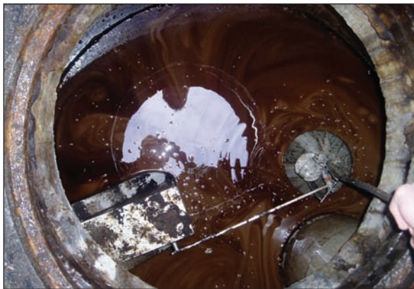
"Closed" valve due to submerged float after diesel oil spill
